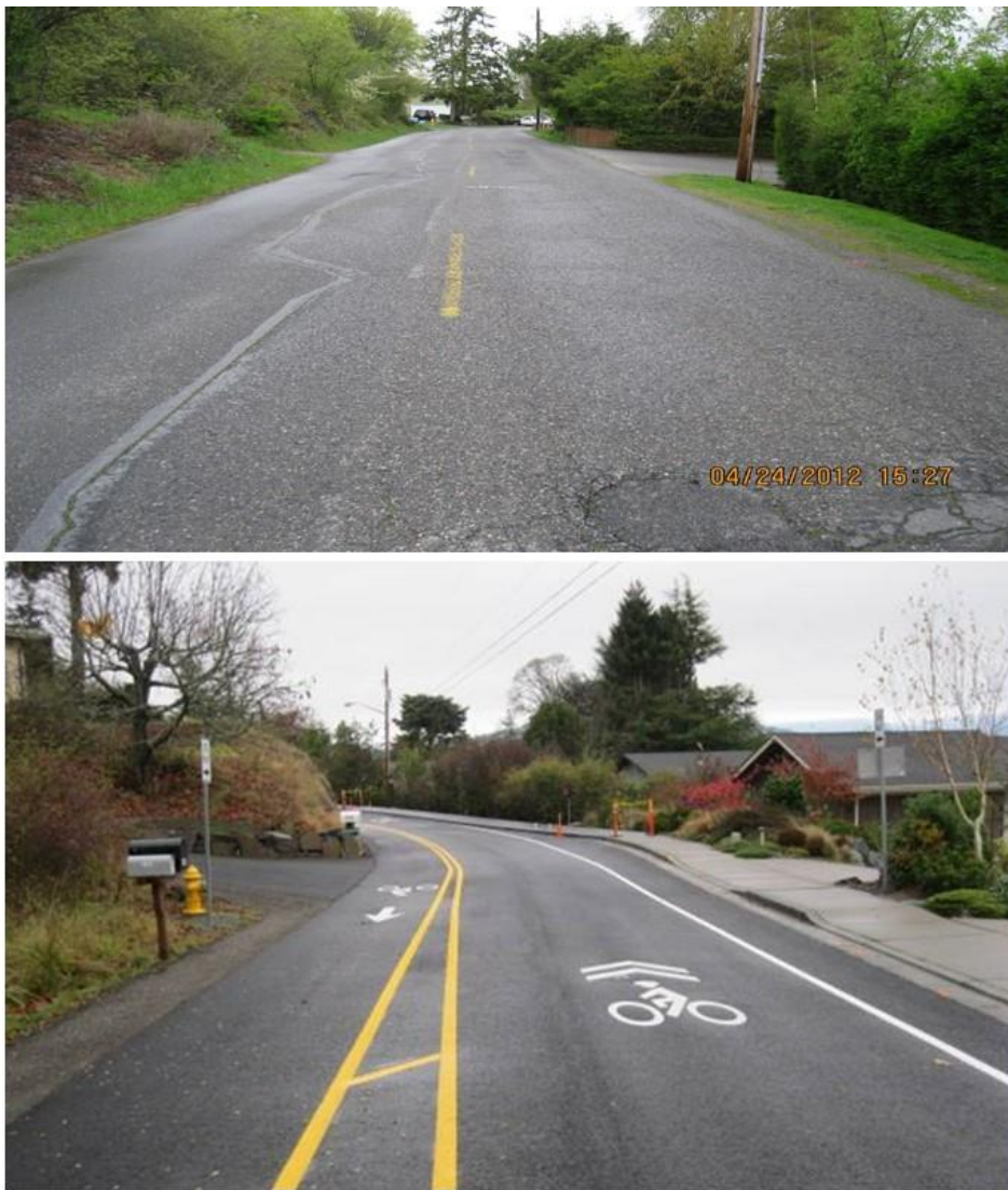
Figure 34. Images above show a before (top) and after (bottom) condition of one street treated as part of the SRTS project.
