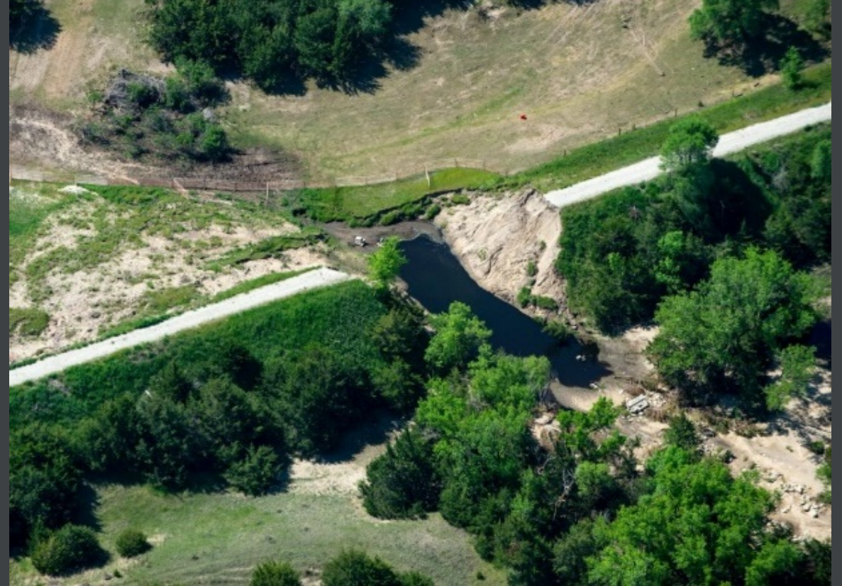
Flood Damage on the Cowboy Trail, Nebraska Image: Outdoor Nebraska Magazine
